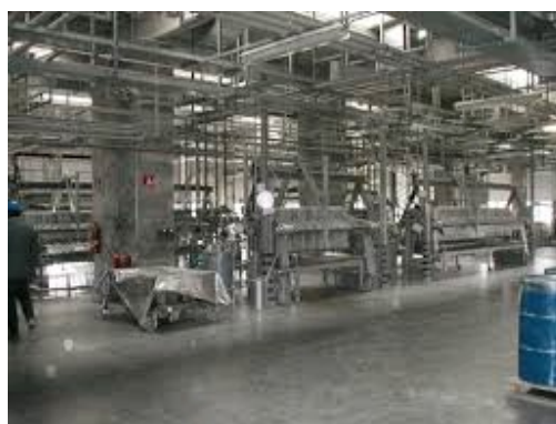
MEPOSA ECKART - RIVANAZZANO (PV)
